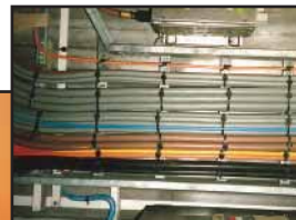
Marine Cable Bundling
